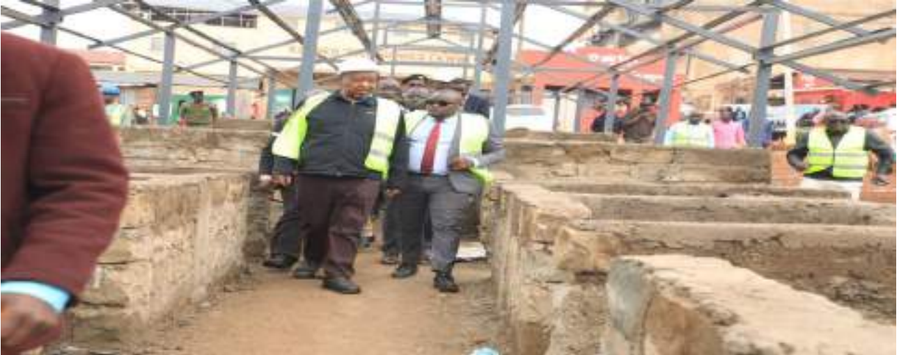
• His excellency the Governor and Rigoma ward MCA inspecting the construction of keroka market stalls
