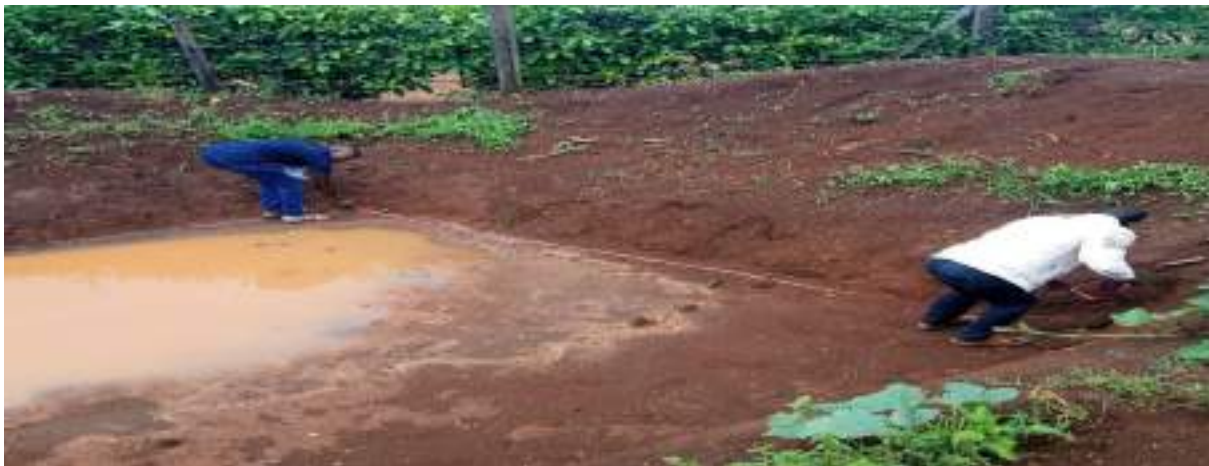
Picture 1.9: showing Nyamira South Subcounty Fisheries officer and his counterpart ward fisheries officer doing pond measurement to determine the size of the liner required to be fitted.
