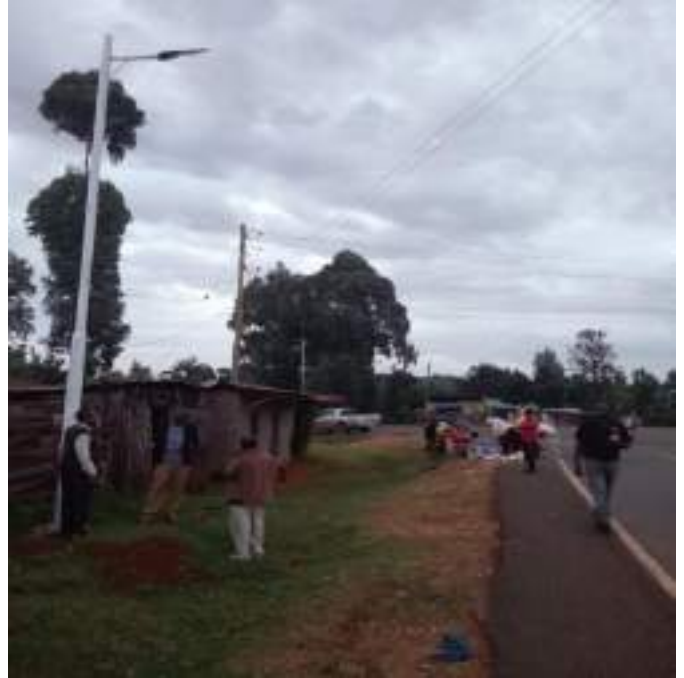
4. Solar Streetlight in Ekerenyo
